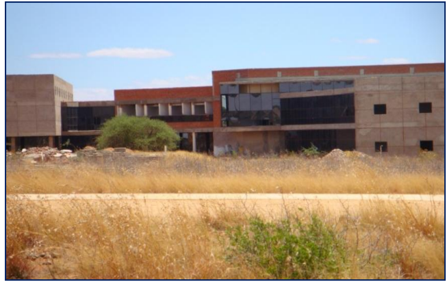
Picture 10: Construction on the New Mental Health Facility that should have been completed during December 2007 was terminated during December 2009 and as at November 2010 the project had not resumed as indicated in the picture.
