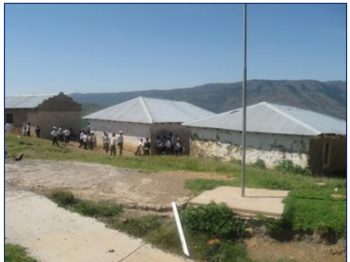
Picture 4: At the Dalindyebo Senior Primary School, learners are taught in two classrooms as indicated in the picture below. Construction of additional classrooms came to a halt during December 2004 and up to July 2011 no further progress has been made.
