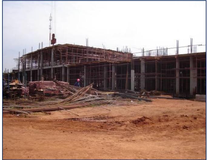
Picture 9: This picture shows the progress with the construction of the Zola Hospital Complex during March 2009, 16 months after the original planned completion date.
